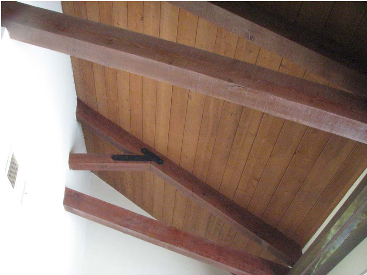
Warring Stone House, roof beams, 837 Park Street, Piru, June 6, 2012 (Charles J. Fisher photo)
