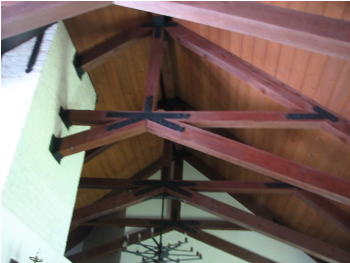
Warring Stone House, living room roof beams, 837 Park Street, Piru, June 6, 2012 (Charles J. Fisher photo)
