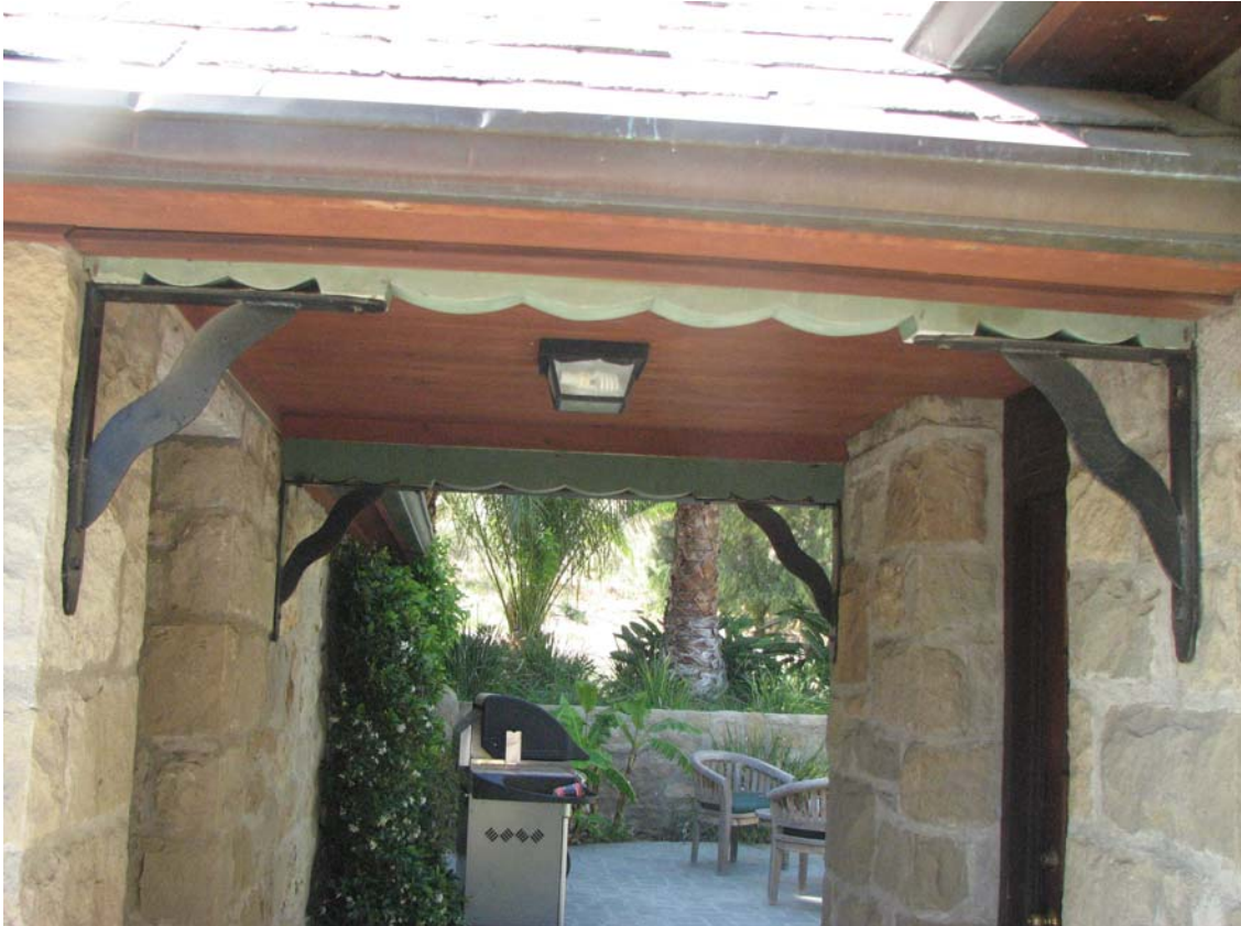
Warring Stone House, roof between house and garage, 837 Park Street, Piru, June 6, 2012 (Charles J. Fisher photo)
