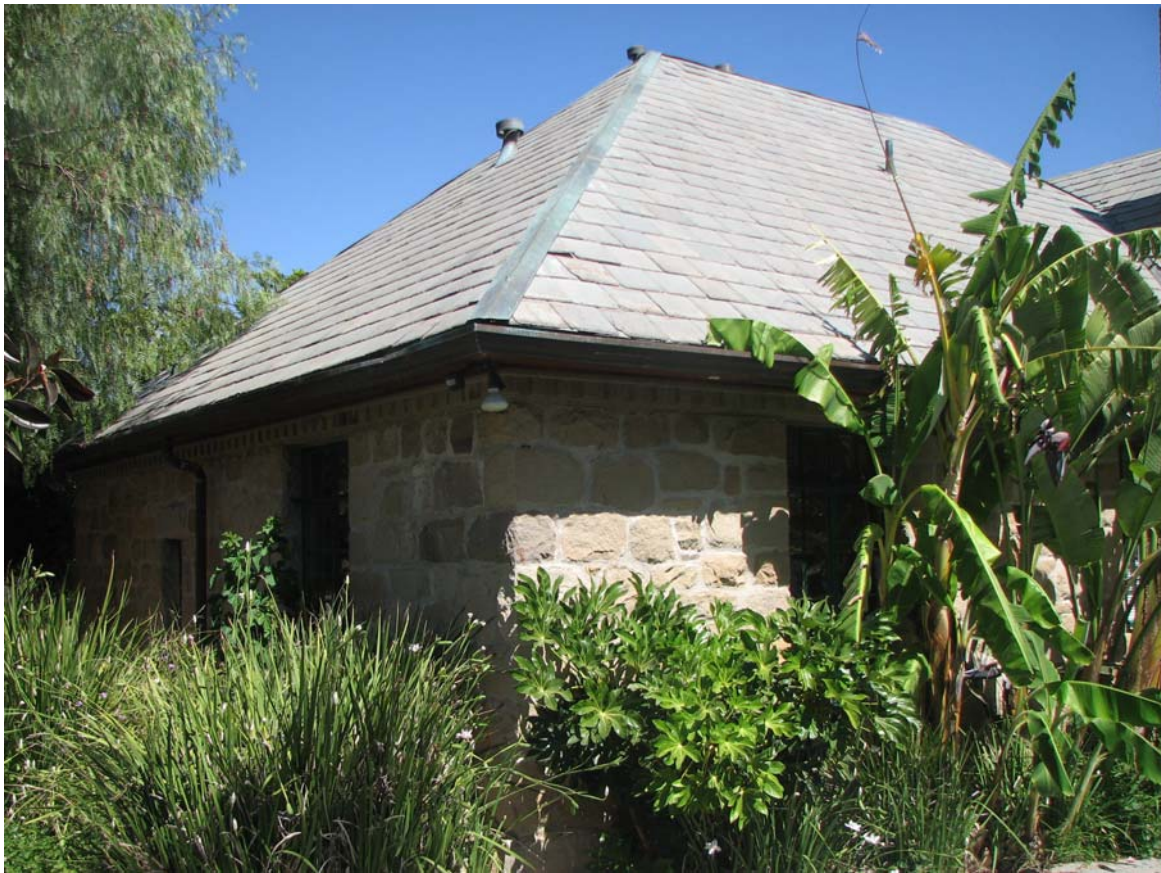
Warring Stone House, slate roof, 837 Park Street, Piru, June 6, 2012 (Charles J. Fisher photo)
