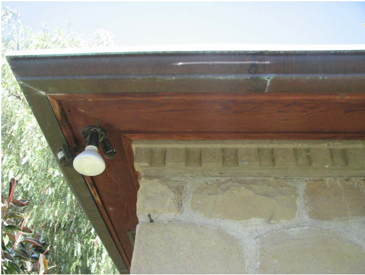
Warring Stone House, closed eaves and dentils, 837 Park Street, Piru, June 6, 2012 (Charles J. Fisher photo)
