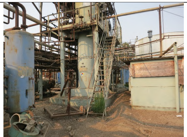
Image 6. Smaller tanks and equipment looking south.
