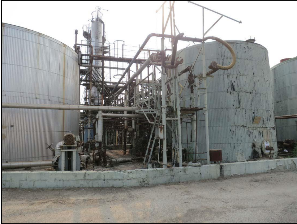
Figure 27. View showing tank 3501 to the left and Tank 1002 to the right, looking east.
