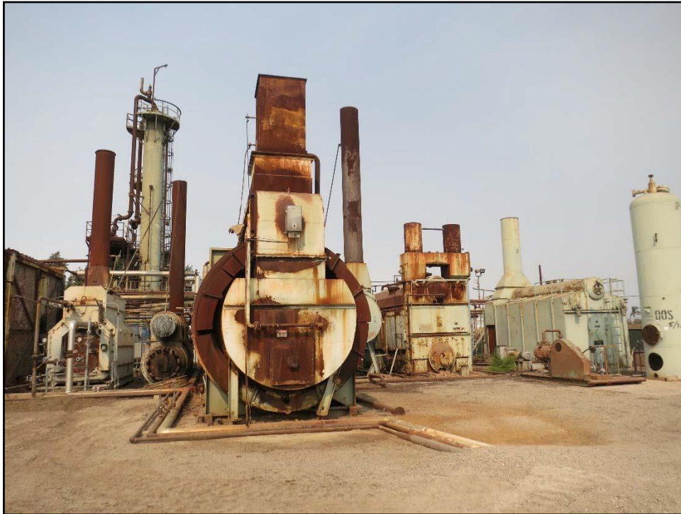
Figure 41. Boilers and other equipment in the Process area, looking west.
