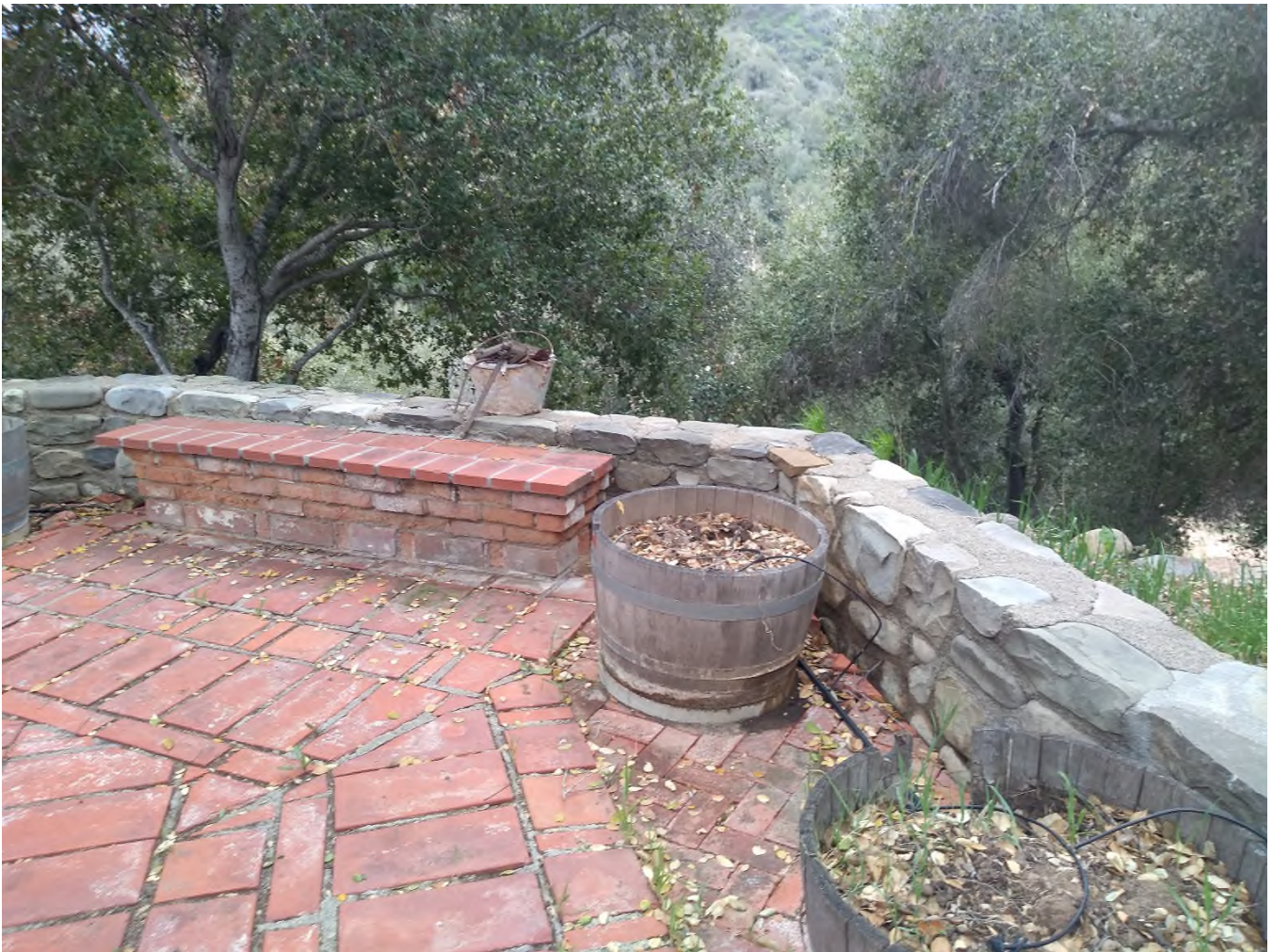
Photograph 36, Rear Terrace, detail of parapet and brick paving, existing conditions, looking south
