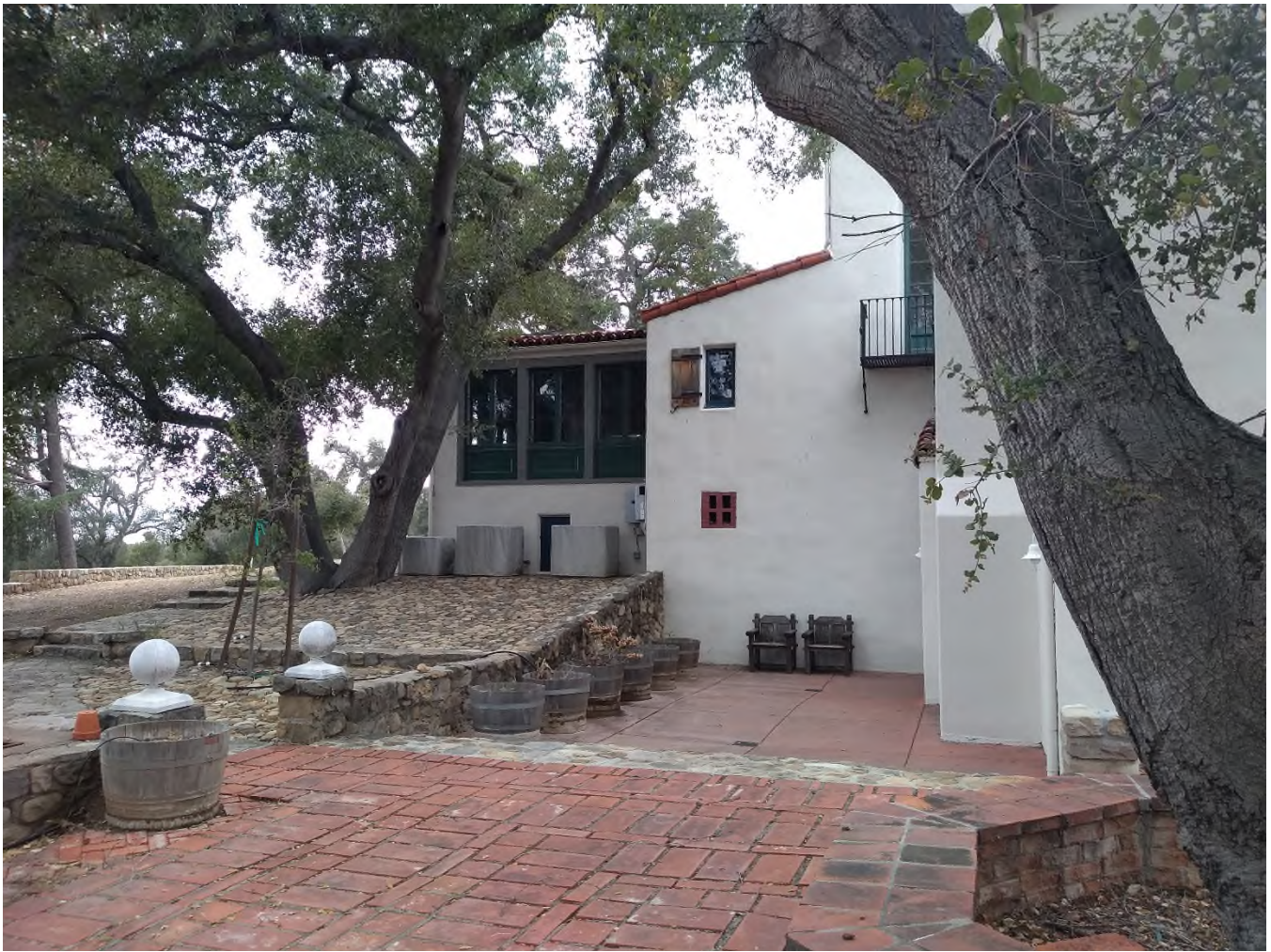
Photograph 13, South Elevation, detail of the west end of the elevation, existing conditions, looking northwest
