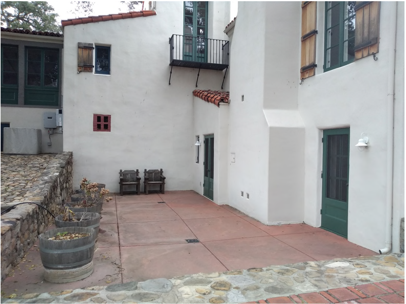
Photograph 14, South Elevation, near west end of elevation, detail of balcony, existing conditions, looking north
