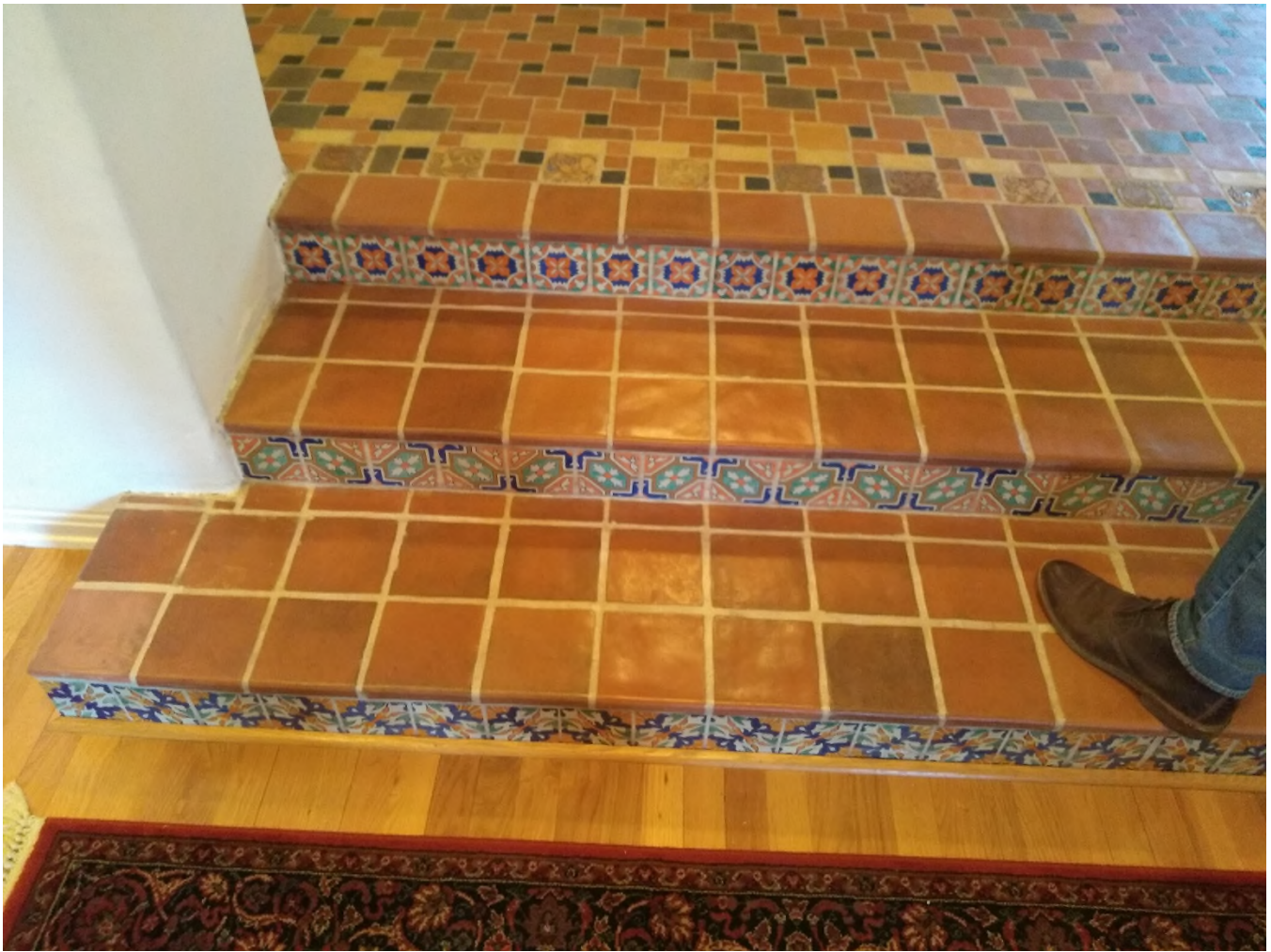
Photograph 20, Entry Hall, detail of stairs to living room, existing conditions. Tilework by Ernest Allan Batchelder and Malibu Potteries
