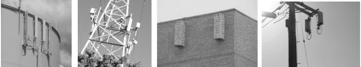
Examples of Flush Mounted Wireless Communication Facilities
