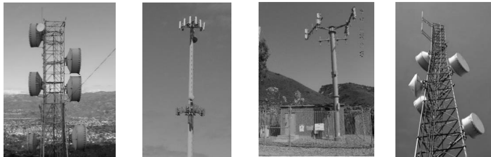
Examples of Non-Stealth Wireless Communication Facilities
