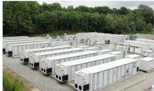
A 50 MW Battery Energy Storage Facility
