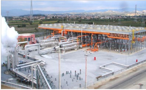
A 50 MW Geothermal Power Plant
