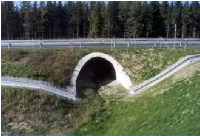
Figure 5.10: Arch culvert with fence for large mammals and lipped wall for amphibians (FHWA/US DOT, 2002)
