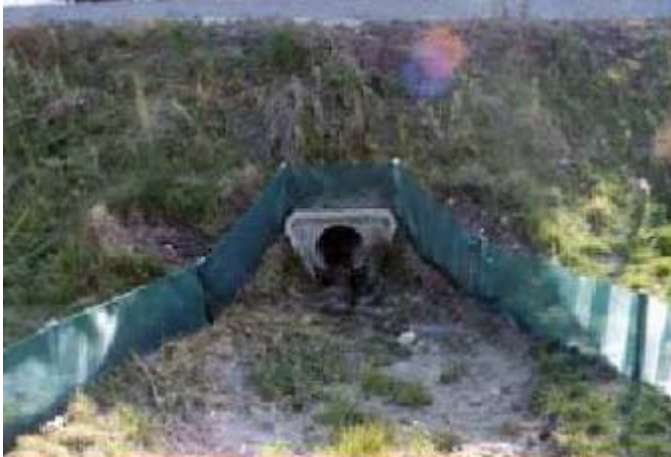
Figure 5.9: Small pipe culvert with mesh fence for small mammals and amphibians (FHWA/US DOT, 2002)
