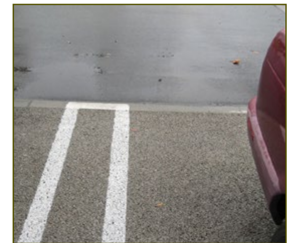
These parking stalls use pervious concrete which allows for water infiltration; the drive aisles are made with traditional asphalt. The County has high expectations for stormwater management in parking areas. Section 8108-5.9
