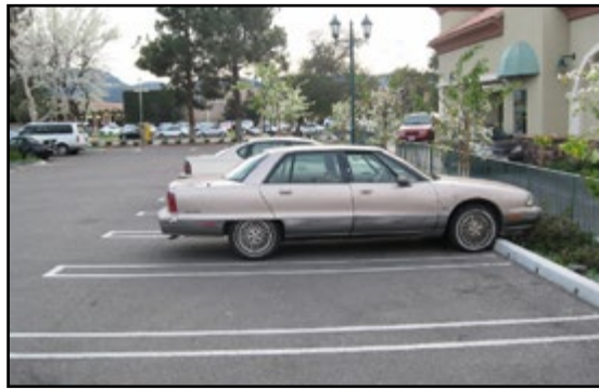
The length of this parking space could be decreased by 2 feet since the parking space allows the car to overhang the landscape planter. Sec. 8108-5.6.3(a)
