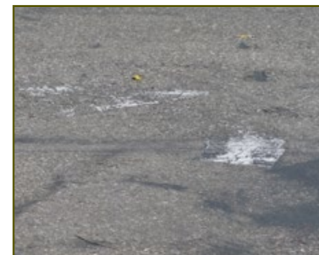
These directional markings have been allowed to fade to the point that they are no longer legible to parking area users.
