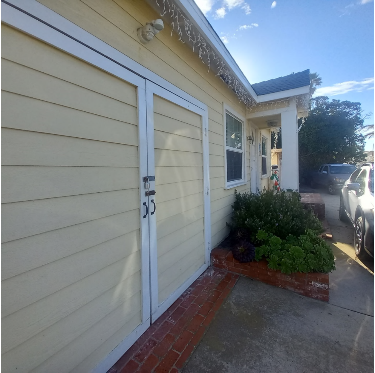
Photograph 13, Looking southwest towards the garage doors on the north elevation of 136 Los Angeles Avenue (December 28, 2023)
