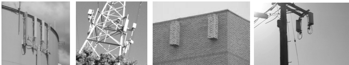
Examples of Flush Mounted Wireless Communication Facilities
