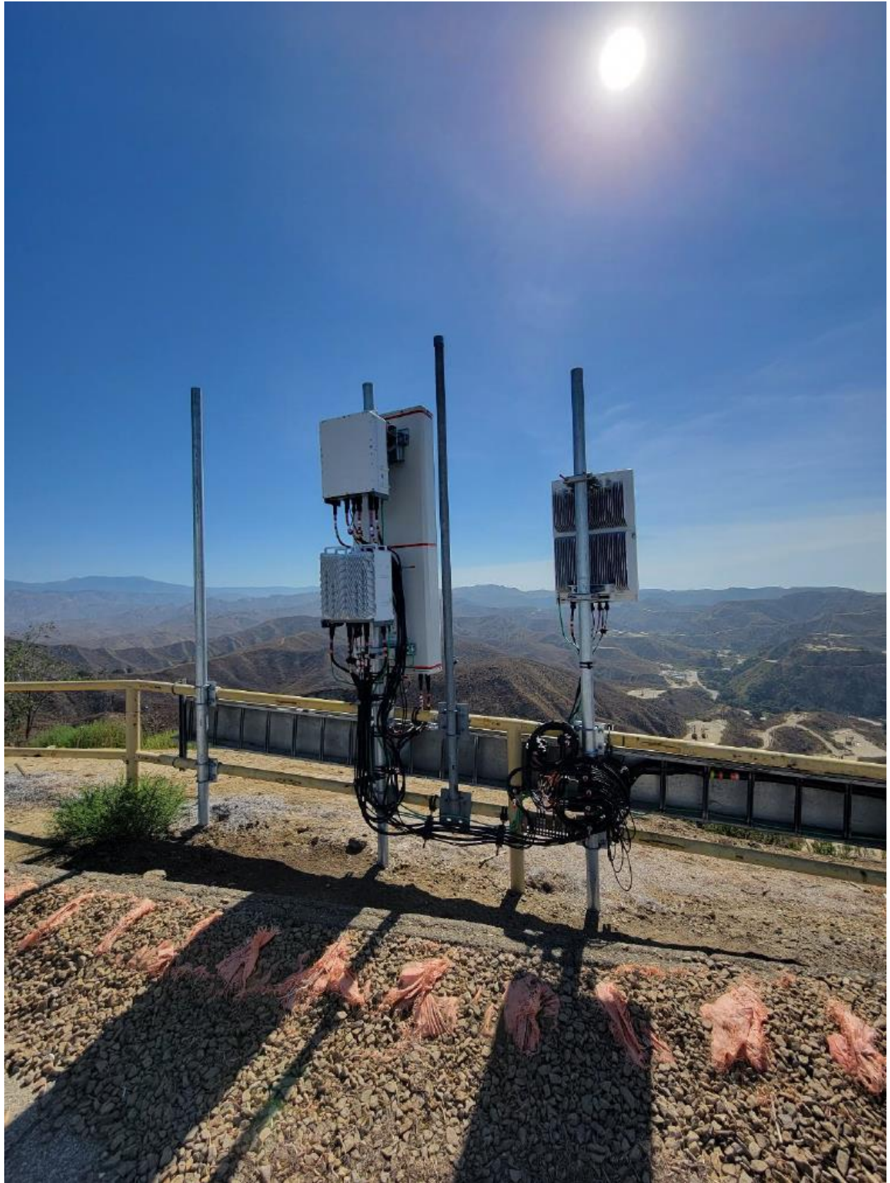
County of Ventura Planning Director Hearing Case No. PL24-0001 Exhibit 5 - Site Photos
