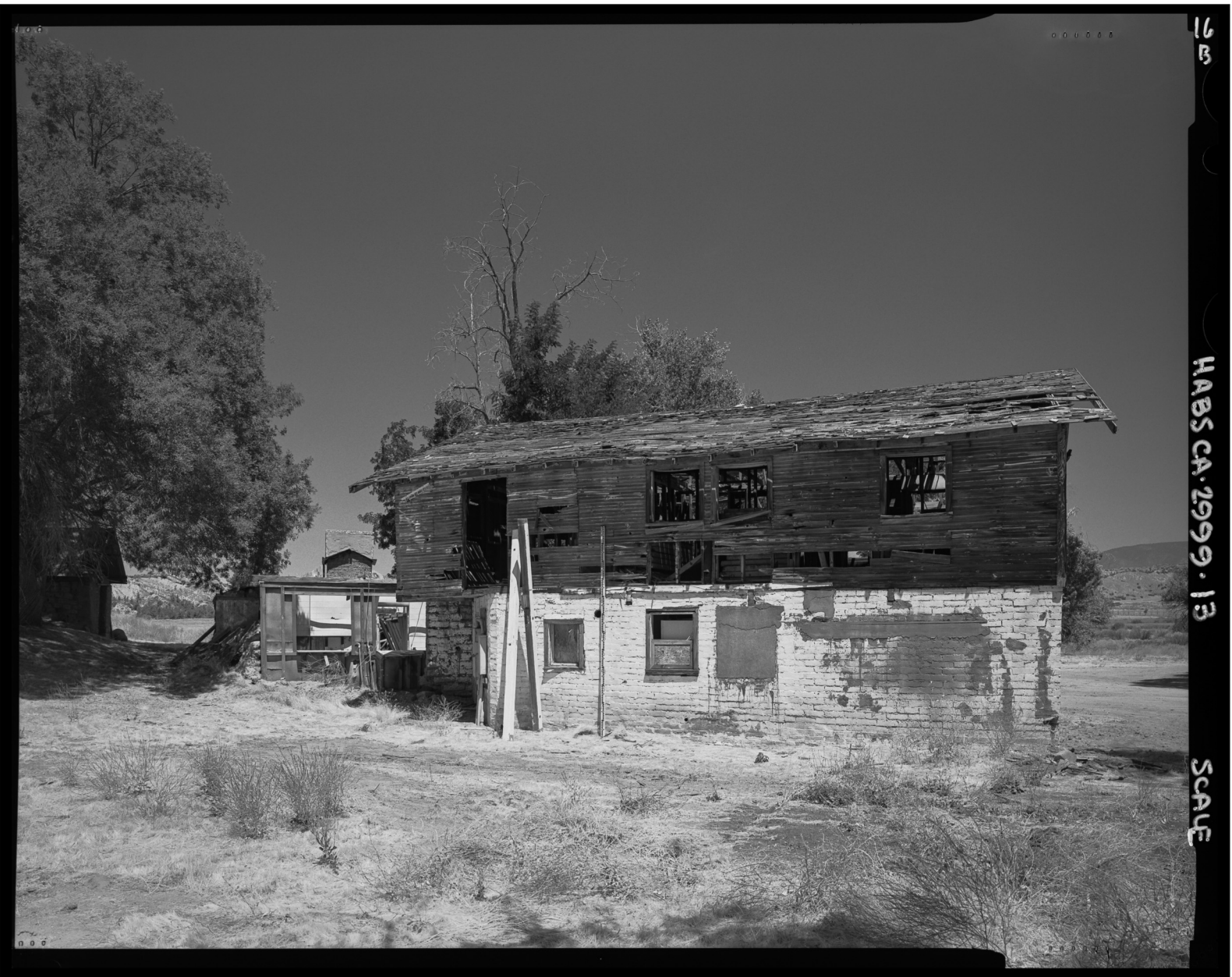
HISTORIC AMERICAN BUILDINGS SURVEY SEE INDEX TO PHOTOGRAPHS FOR CAPTION HABS No. CA - 2999 - 13
