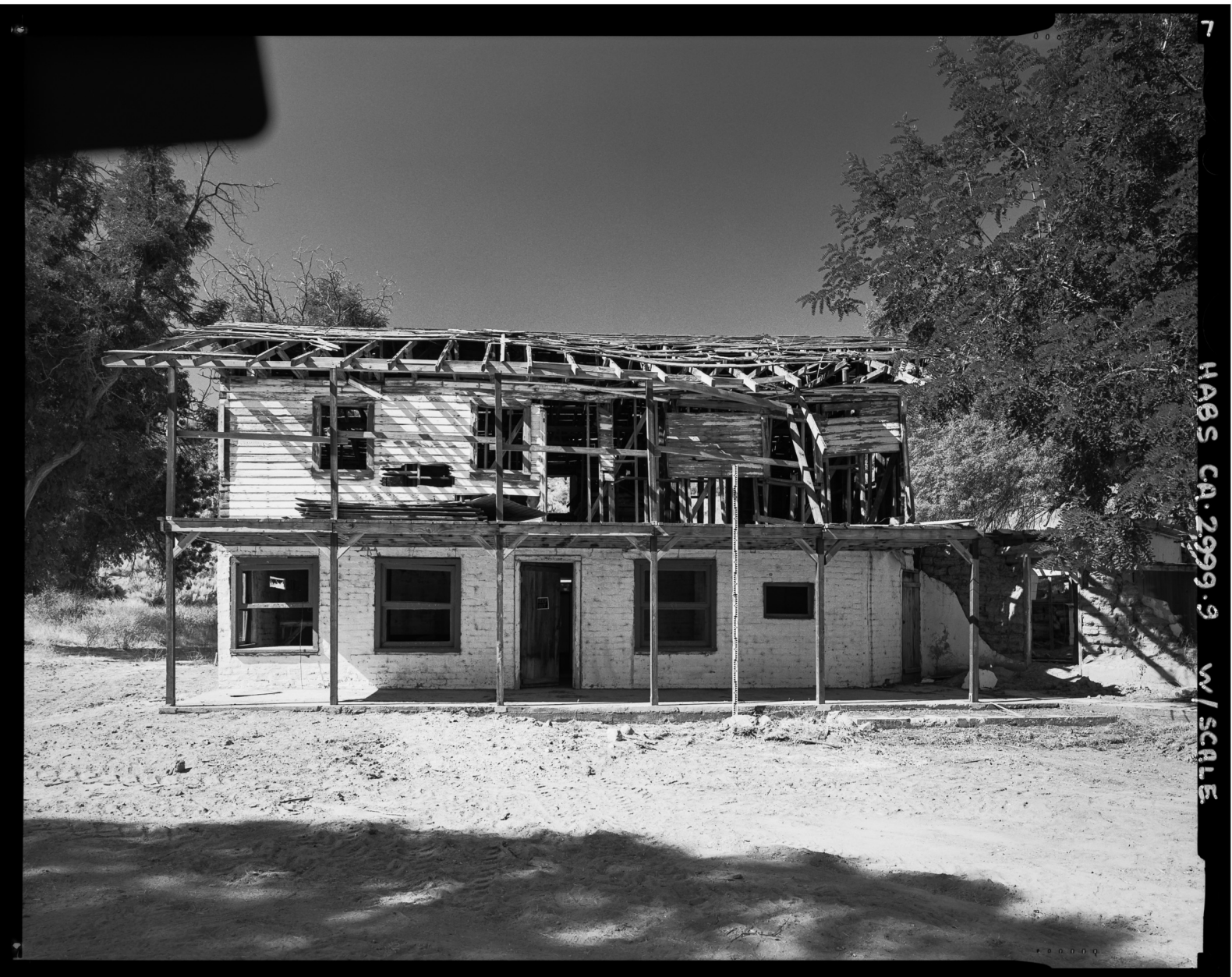
HISTORIC AMERICAN BUILDINGS SURVEY SEE INDEX TO PHOTOGRAPHS FOR CAPTION HABS No. CA - 2999 - 9
