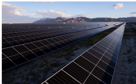
A 50 MW Solar Photovoltaic Array Ocotillo Wells Solar, Borrego Springs, CA Approximately 336 acres
