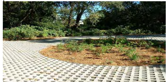
Grass pavers allow infiltration of stormwater while providing a load-bearing surface. This picture shows the project in the final stages of completion. The voids between the concrete lattice structure should be filled with a loamy material to allow for sufficient infiltration rates.
