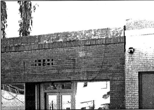
A concrete parapet rests atop a soldier course of brick on a shop building in Piru's unique Commercial Town Center.
